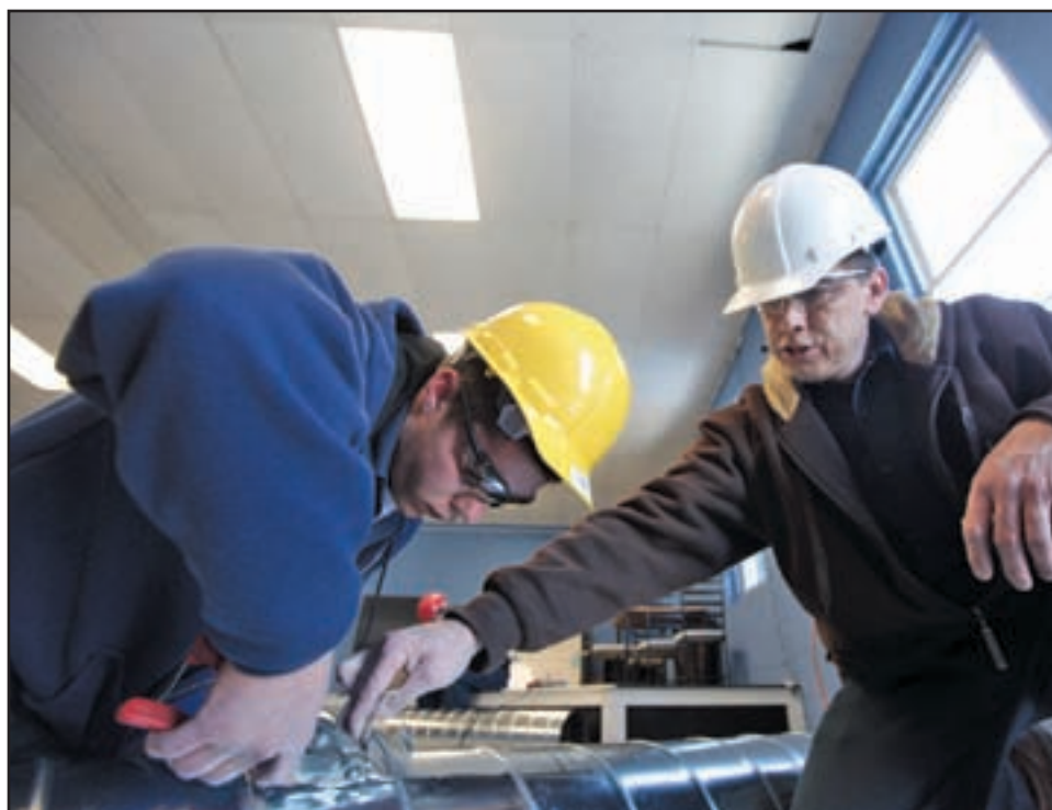
ON THE JOB TRAINING Sean Mulkern (right), an HVAC instructor at the South Shore Vocational Technical High School with student Connor Clancy. Mulkern became a teacher after spending 30 years in the HVAC field.
